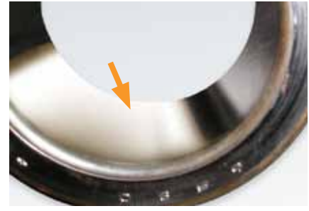
Cone bore polishing: Contact wear/creeping on the shaft, with no lubrication between the cone bore and shaft OD, caused by cone bore contraction resulting from excessive tight setting (preload).
